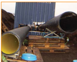
20 foot sea container used as a dry and secure housing
